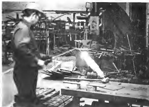
Blacksmith-welder John Rebacz heats the center of a fish plate (on bricks) to a cherry red color (about 1800° F) with a torch.
