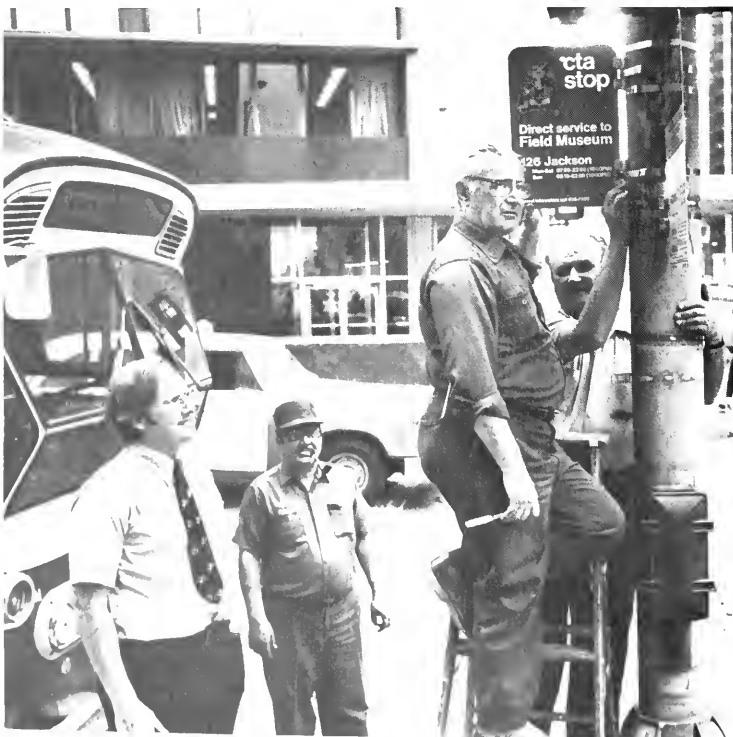
Shown installing special King Tut bus stop signs along the No. 126 Jackson route are, from left to right, Bob Grady, planning technician; Bill Brandon, service truck driver; Al Guadagno and Larry Girlich. Pictures were made at Jackson and Warner drive.
