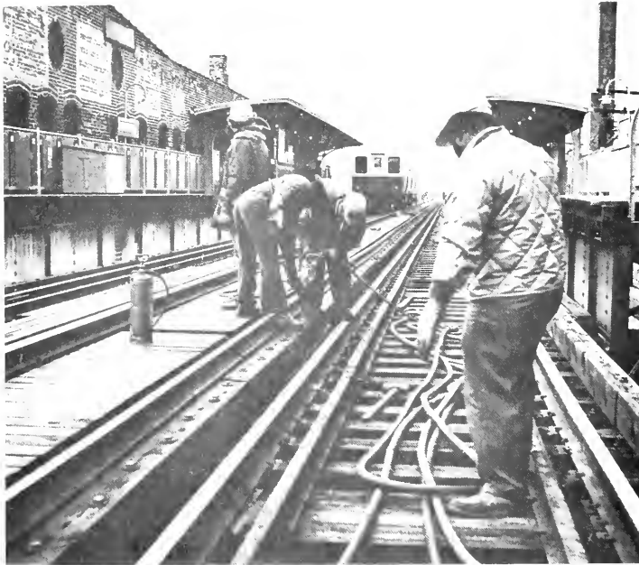
ON THE TRACK: The Track Department has four structure gangs working on major track renewals on the Ravenswood, Douglas and North-South routes. The work is part of the capital improvement program.
