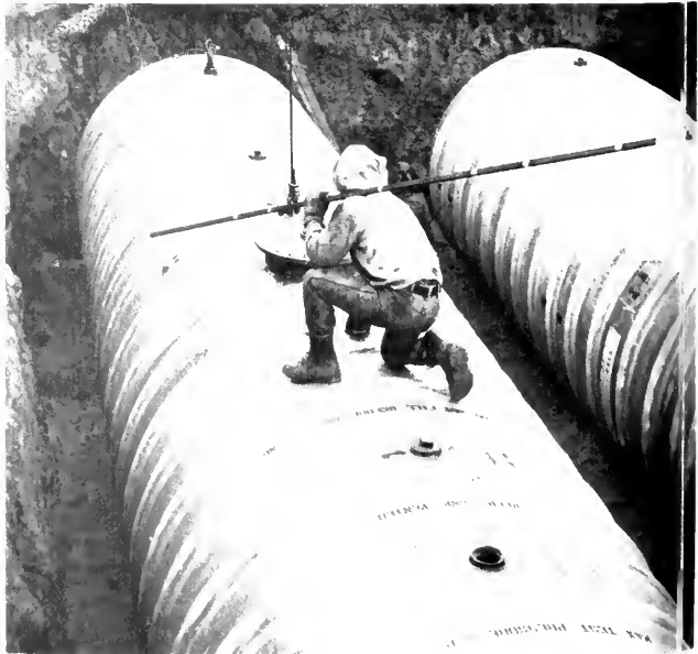
FUEL CAPACITY INCREASED: These two new tanks (holding more than 10,000 gallons each) have been installed at CTA's Archer garage. They replace smaller tanks. The new larger tanks permit a reserve of sufficient fuel to sustain a three day holiday weekend of service by 252 buses running regular service out of Archer.
