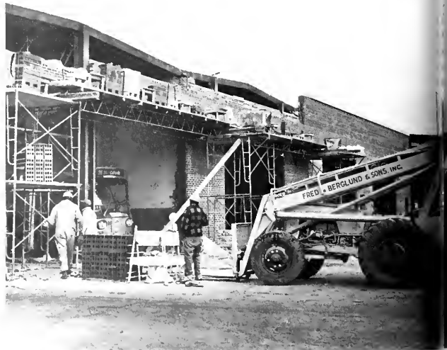
ARCHER DOOR PROJECT: Other renewal work at Archer garage includes widening of doors, here shown under construction. Renovation of the doors, originally designed for streetcars, will reduce repair costs. Project, which is on schedule, will be completed in late summer of '77.
