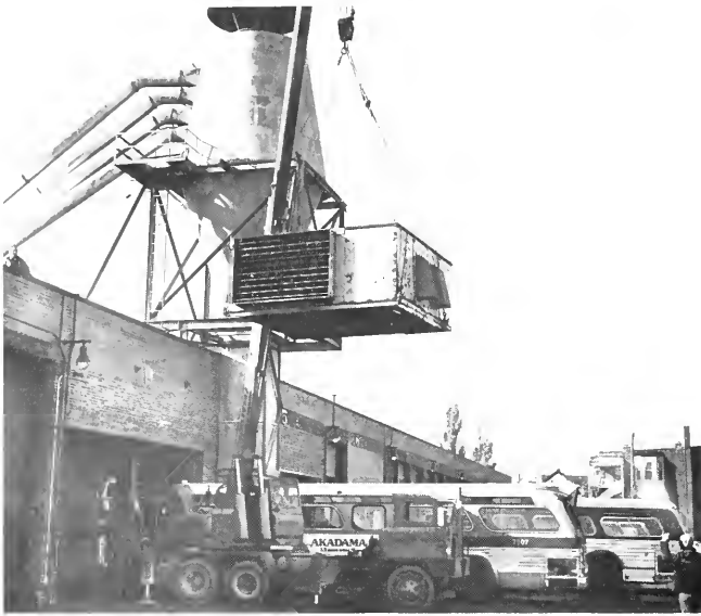
HEAT TO THE ROOF: Swing to the roof of the Archer garage is the first of two new heaters with a 2.5 million BTU capacity per unit. The new units replace two smaller heaters which had been used for 10 years. Steel structure of the building was altered to accommodate the larger units and new wiring was installed. The $400,000 project also includes improved heating in the bus fueling and washing bays.
