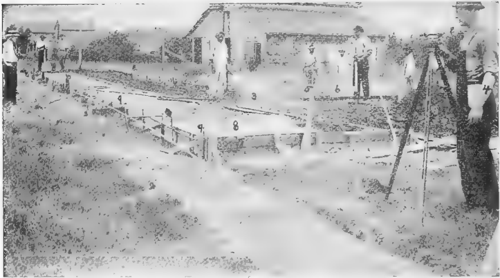
FIG. 83.—Construction of the foundation and floor. 1, The cinders, which are being leveled and tamped (2) after being wet down (3); 4 is the survey outfit to find the level; 5, mixing the concrete; 7, the forms which extend 1 foot into the ground and in which the 4-inch concrete wall is made; 8, the 3-inch coat of coarse concrete; 9, the bolts set into the concrete to which the 4 by 4 inch sills are to be bolted.
