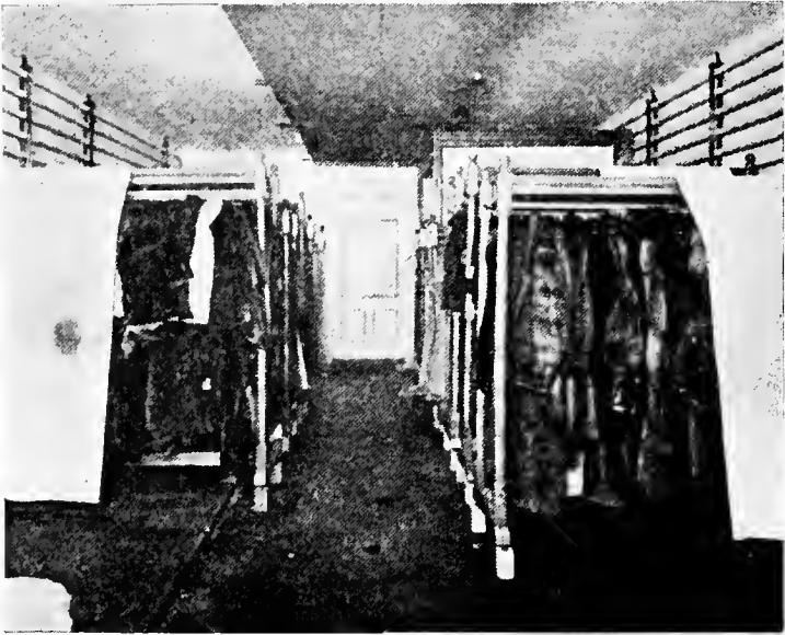
FIG. 9.—COLD STORAGE ROOM FOR GARMENTS, SHOWING PIPING.
