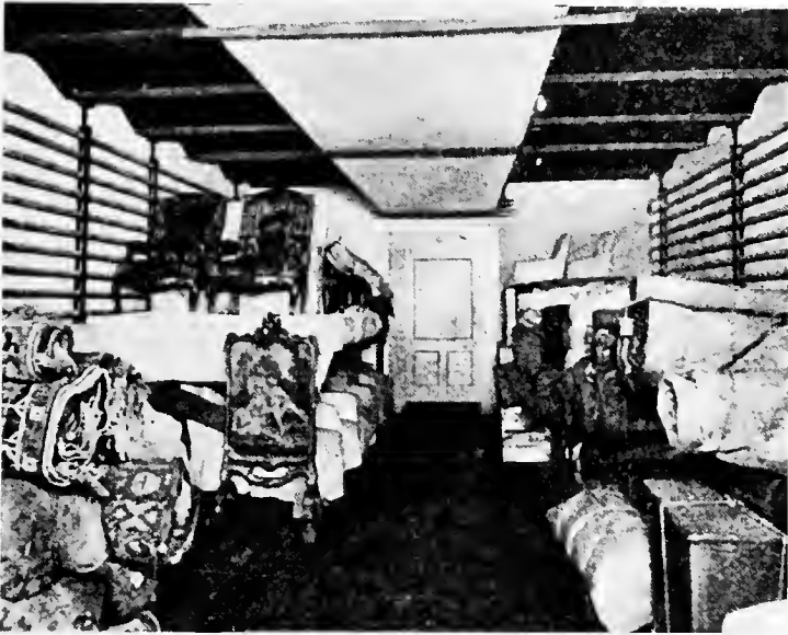
FIG. 10.—COLD STORAGE ROOM FOR CARPETS, SHOWING PIPING.
