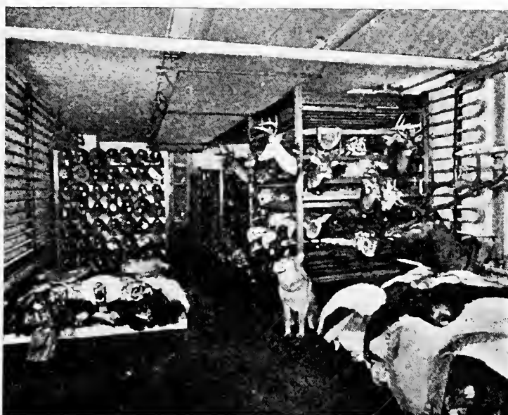
FIG. 8.—COLD STORAGE ROOM FOR FURS, SHOWING PIPING ON SIDE WALLS.
