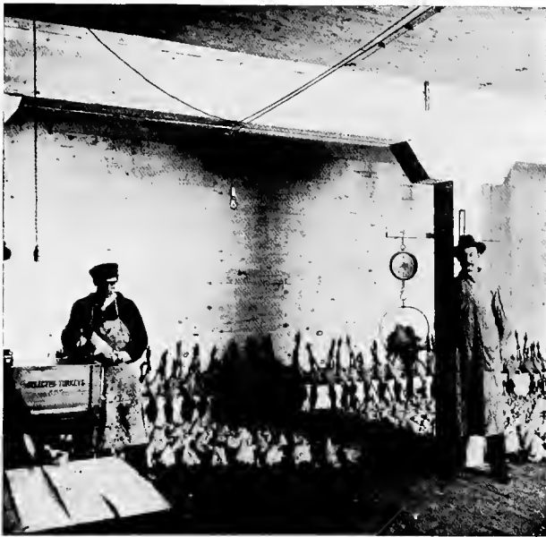
FIG. 5—COOLING POULTRY IN A ROOM EQUIPPED WITH COOPER FALSE FLOOR AND FALSE CEILING SYSTEM OF AIR CIRCULATION.
