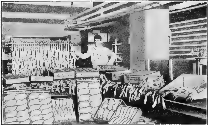
Figure 3.—Interior view of a modern cold-storage plant.
