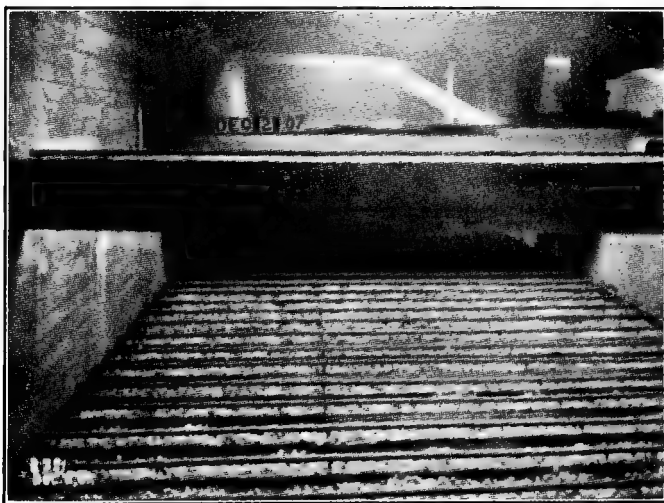
FIG. 102.—One of the ten filter beds of the Columbus water filtration plant with the filtering material removed. Sand is the filtering material. All of the beds together have a capacity of 30,000,000 gallons daily.
