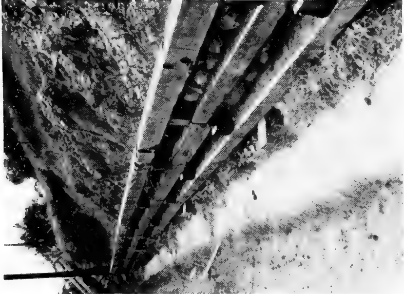
Reinforced thin concrete lining of a roadside ditch, and support of sliding toe of hill with
