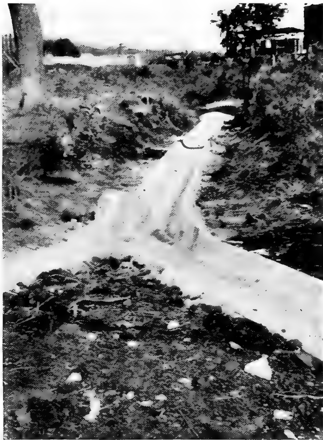
Junction of concrete ditches, showing splash wall to confine water within the ditch
