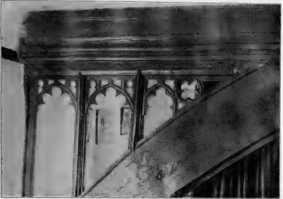
LITTLE HADHAM : CLINTONS, BURY GREEN : ROOF SPANDEL IN BEDROOM
