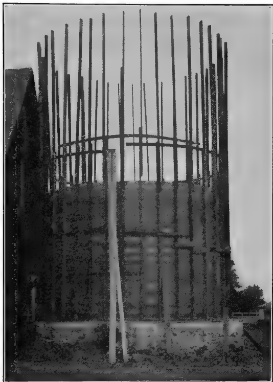
FIG. 88.—SILO IN THE PROCESS OF CONSTRUCTION BY FARM LABOR. This silo, 16 feet in diameter and 30 feet high, was completed at a cost of one dollar for each ton capacity.
