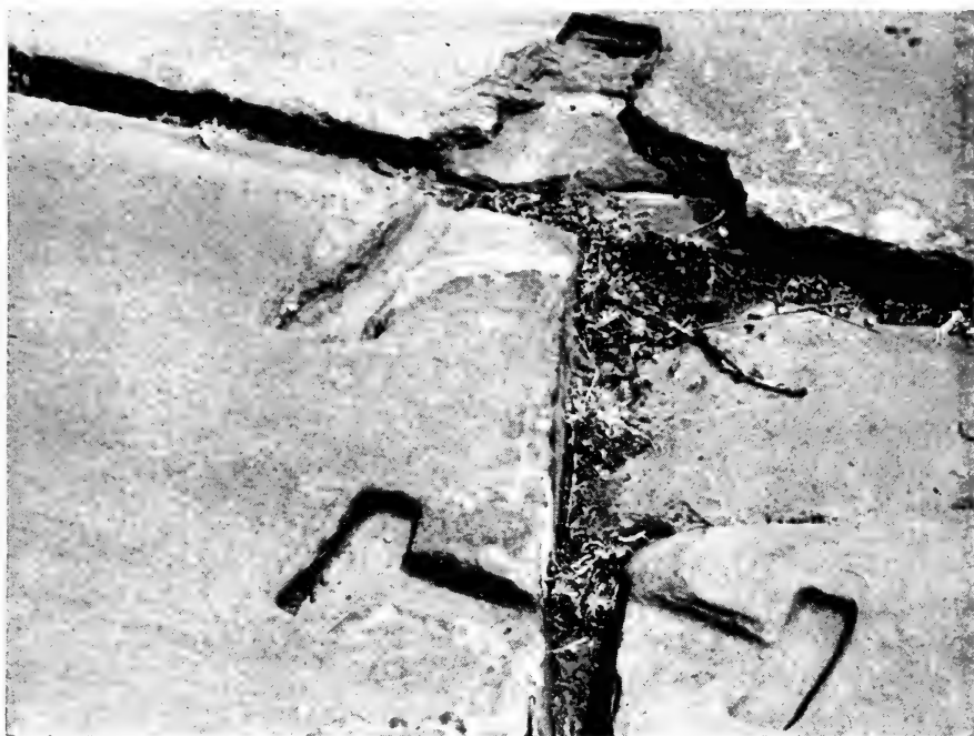
FIG. 38. Typical wall construction and detail of sockets for cast copper cramps or tie bolts in stone paving at Tialuanaco.
