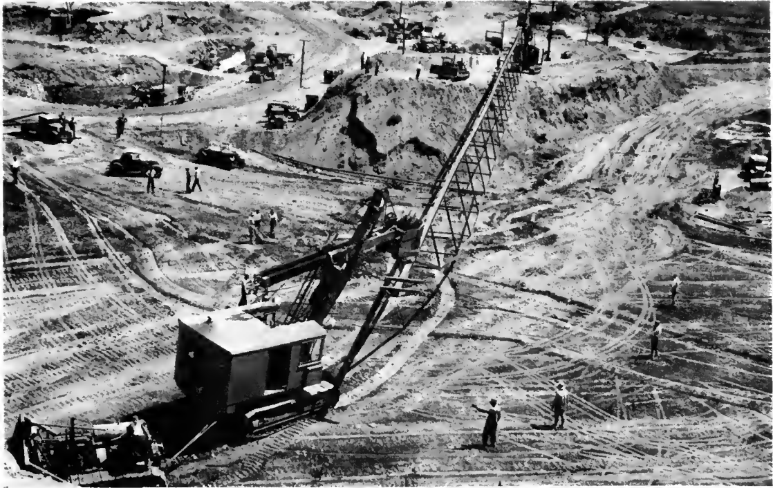
The photograph above shows another view of equipment utilized in the construction of Santiago Creek Dam.
