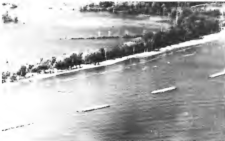
Figure 15. Prototype test breakwater at East Harbor State Park, Ohio sediment has built up behind the breakwater and the local bathymetry is beginning to show subaqueous evidence of salient development. The state of Ohio is currently monitoring this project.
