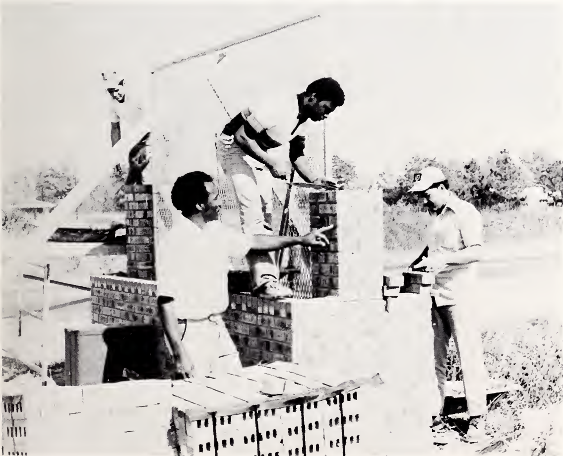
Masonry students, Herbert Oxendine, Moses McDuffie, and Billy Jacobs, receive directions from their instructor, Mr. Collie Brown, as they work on the welcome sign that they built for the Town of Pembroke.
