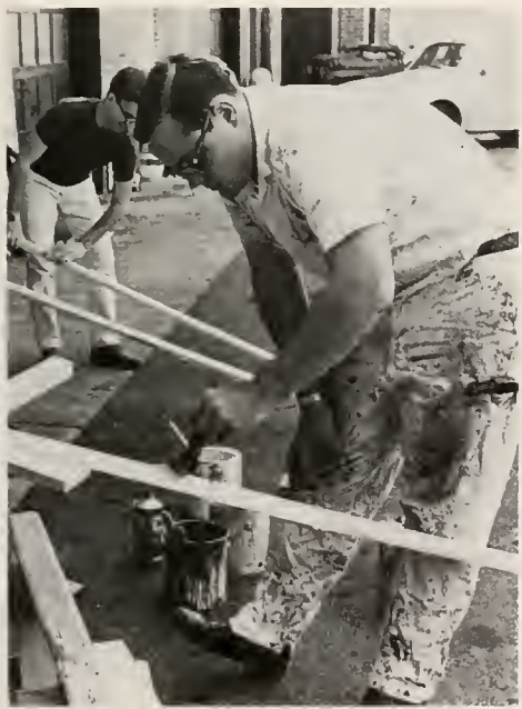
Tom Mowbray paints wooden slats to be used in the repair of campus benches.
