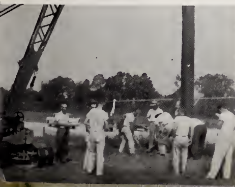
Lights For The Football Field.
