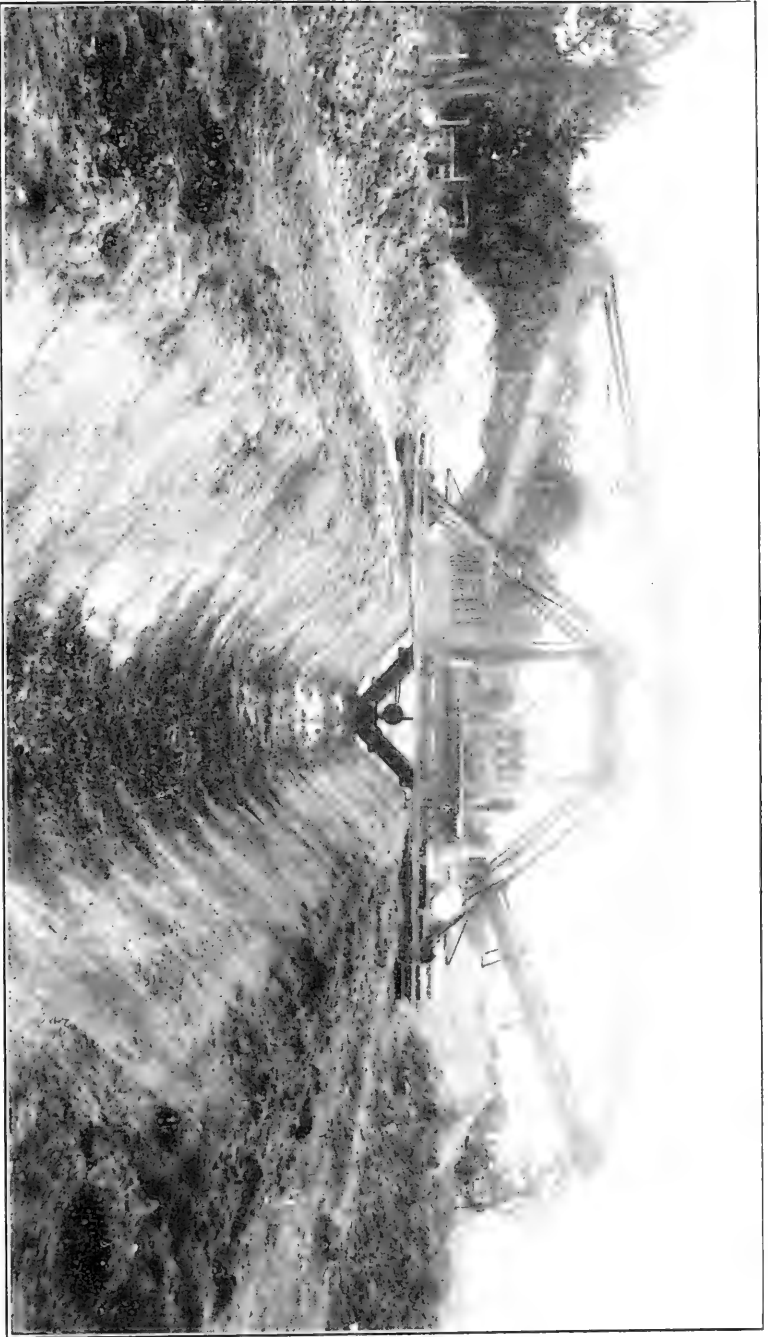
Fig. 9. A Dry Land Dredge or Excavator Constructing a Narrow Bottom Drainage Ditch.
