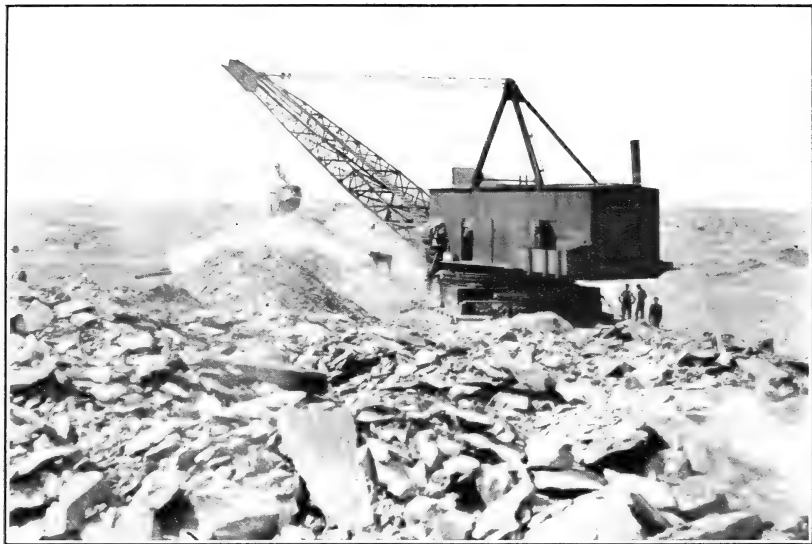
FIG. 1.—PRESSURE HAS CAUSED SHEARING ALONG BEDDING PLANES; WHEN EXCAVATED THE SHALE COMES OUT IN LARGE FLAKELIKE PIECES.
