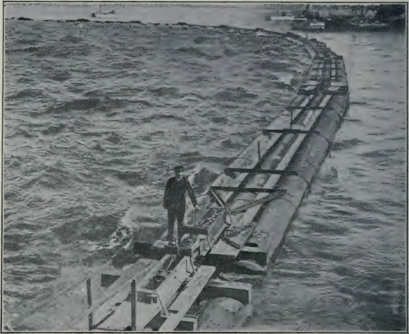
FIG. 36.—Floating Discharge Pipe of the Dredge "J. Israel Tarte."
