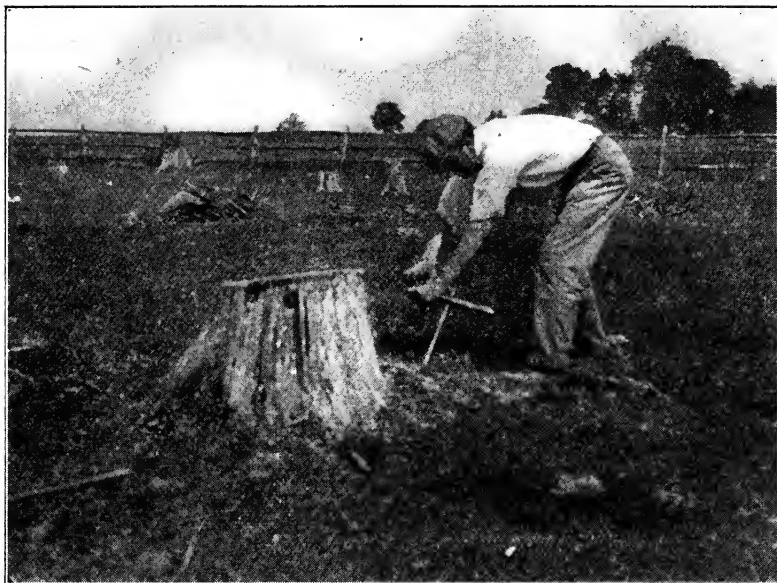
FIG. 12.—BORING HOLE UNDER STUMP WITH DIRT AUGER. THIS IS NOW USUALLY DONE WITH A PUNCH BAR
