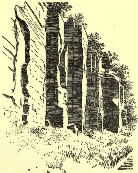
FIG. 36. — A set of master joints developed in shale upon the shores of Cayuga Lake near Ithaca, New York (after U. S. G. S.).
