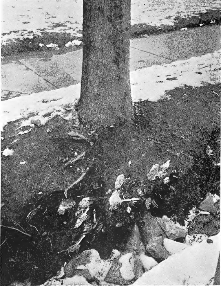
The base of a Norway maple some 18 inches in diameter showing the numerous roots cut when digging a ditch for the installation of a curb. The edge of the ditch is within 9 inches of the base of the trunk of the tree. The Dale Street trees (Plate 7) were probably weakened earlier in a similar manner
