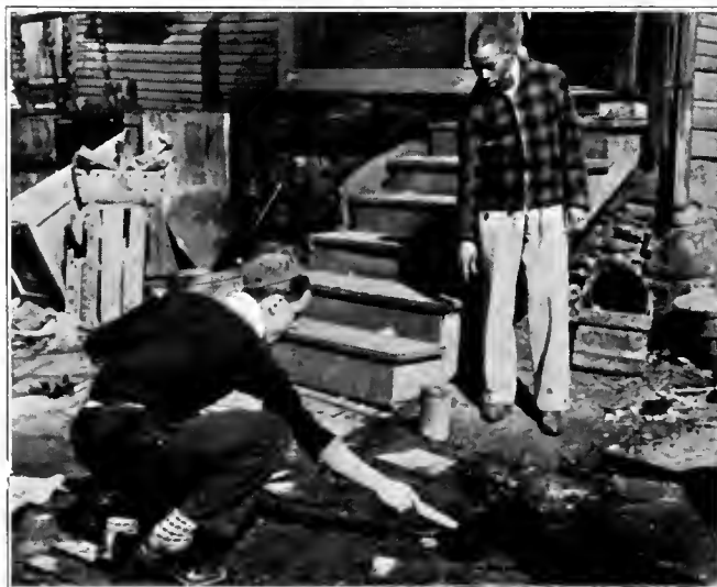
At left—Rear of tenement to be demolished, showing outdoor privy and goods of last family to evacuate building.
