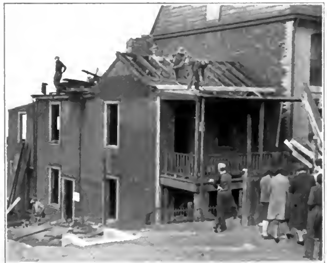
Junior High School pupils viewing demolition of dwelling in preparation for housing project.
