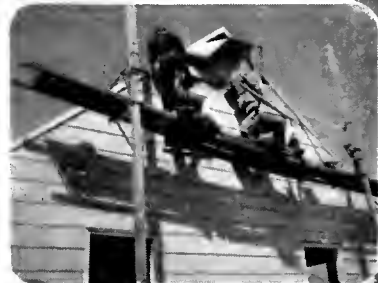
BUILDING A HOUSE. The actual construction of a home is presented so skillfully in this EBFilm that very small youngsters easily get a clear idea of this complicated process. Related EBFilms for your library: Making Shoes; Making Cotton Clothing; Paper; Cotton; Making Books.
