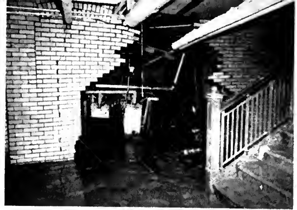
Pressure bursts windows and doors: demolishes two interior walls.
