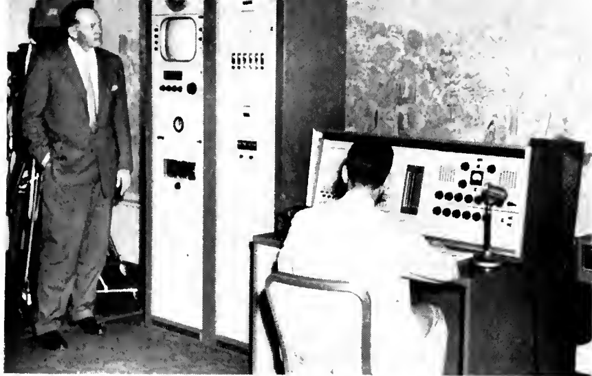
Figure 7. This system (DuKane Co.) incorporates central sound, intercom, fire sensing alarm and other accessories.
