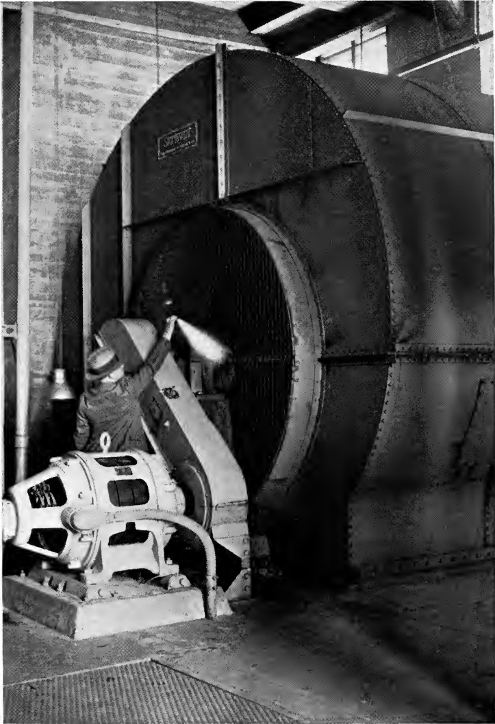
ONE OF THE 84 STURTEVANT SILENTVANE FANS Which are the lungs of the Holland Tunnel
