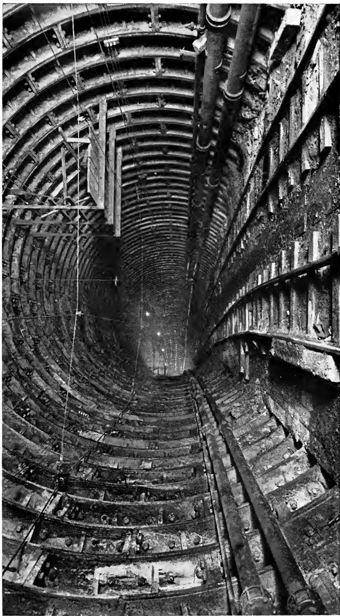
CURVE IN SOUTH TUNNEL UNDER WEST STREET, NEW YORK CITY (RADIUS 1000 FEET) Showing completed rings of cast-iron lining
