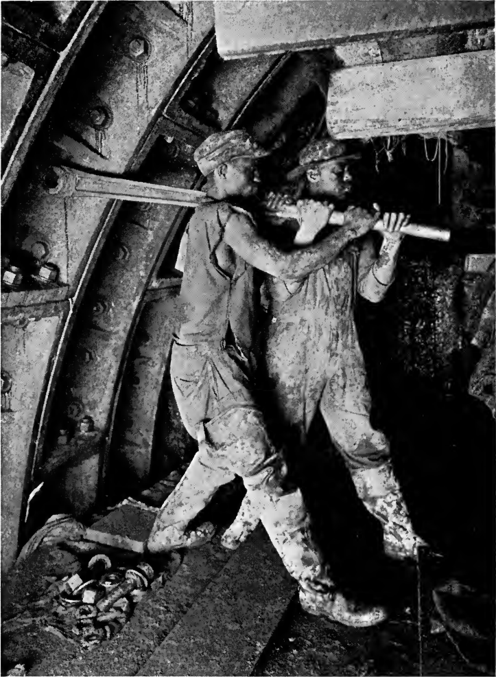
TIGHTENING BOLTS IN TUNNEL LINING, NORTH TUNNEL By means of ratchet wrench. Each bolt weighs ten pounds
