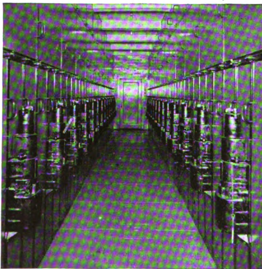
OIL CIRCUIT-BREAKER AISLE
