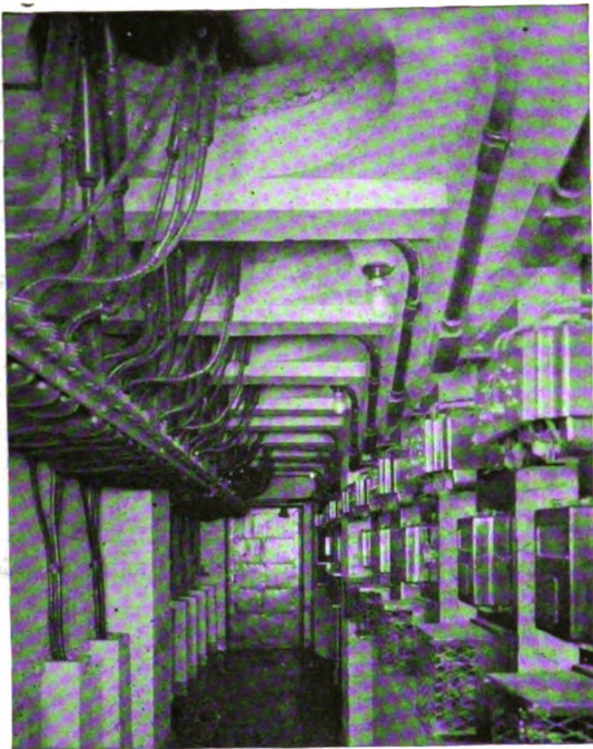
COMPARTMENT BELOW THE INDUCTION REGULATORS
