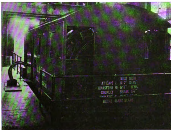
PORTABLE SUBSTATION READY FOR OPERATION
