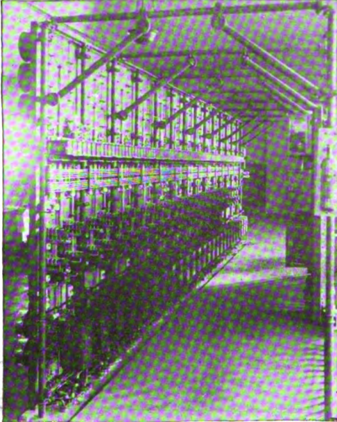
Rear View of Main 13,200-Volt Feeder Board Showing Graphic Meter Panels to rear.
