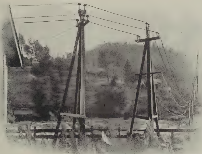
An Angle in One of the High Tension Lines.
