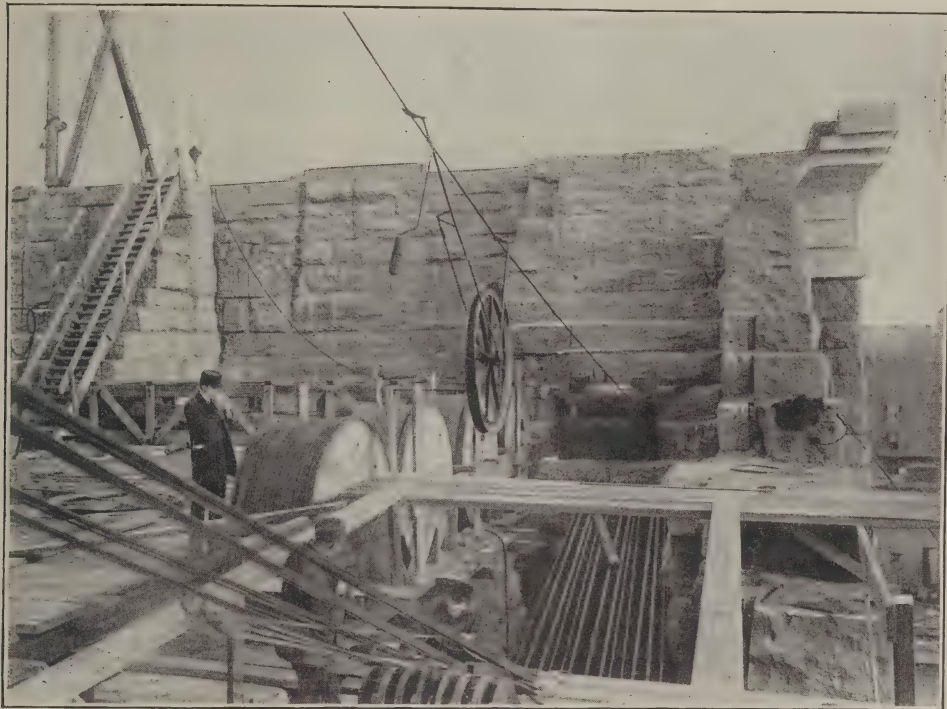
Partial View of a Pier, Showing the Anchorage and the Traveling Wheel.
