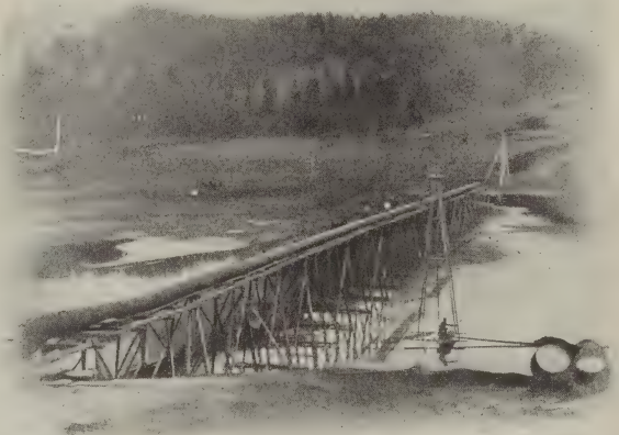
Lake Francis Dam. Dirt Filling Is Washed into the Dam by a Pipe on Falsework Above.
