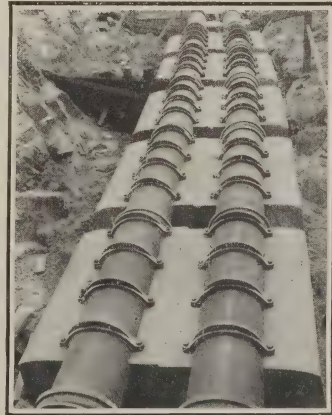
Concrete Anchorage Piers for the Water Pipes.
