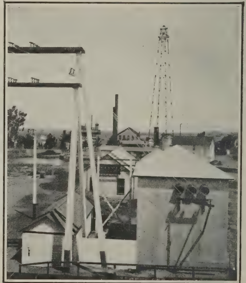
Redwood City Substation and River Crossing.
