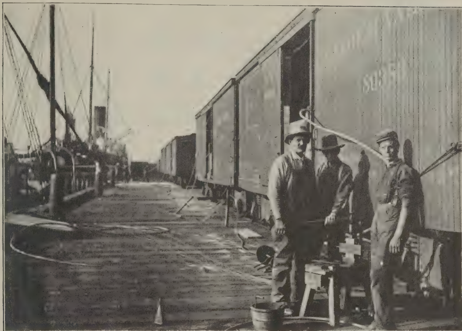
Splicing the Cables in Car-Lengths of 15 Miles Each on the Seattle Wharf
