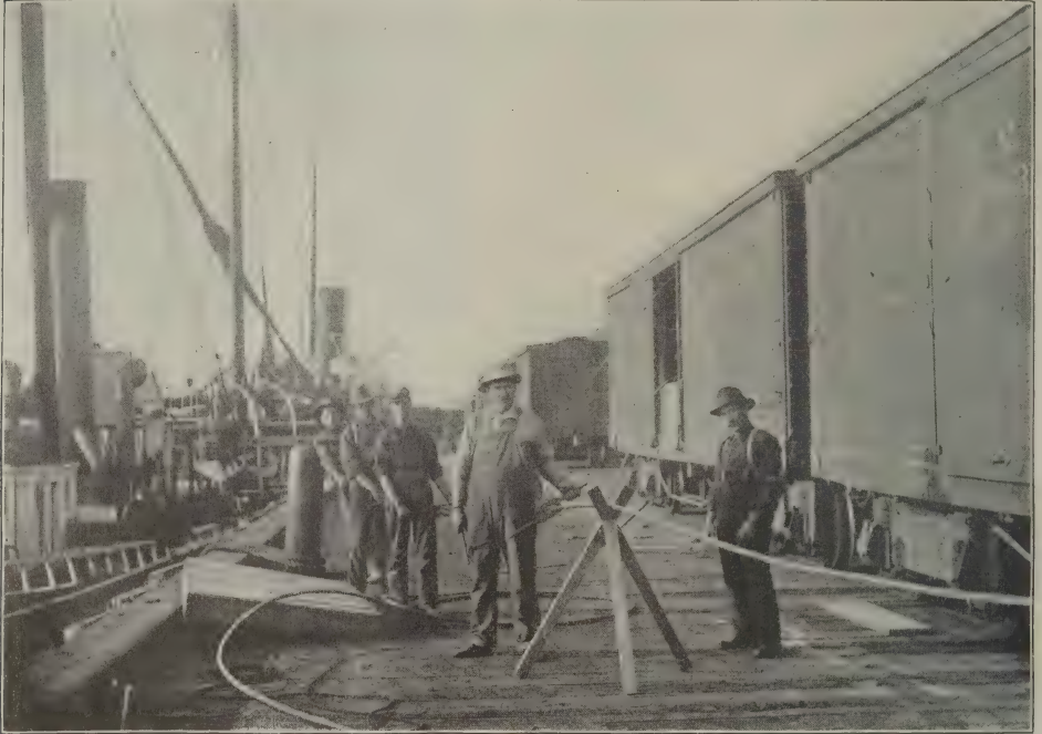
Hauling Cable out of the Cars and Coiling Down into the Lakme's Tank.
