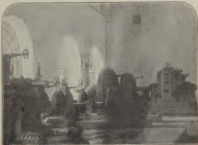
A Glimpse of the Generator Room of the Livet Power House.
