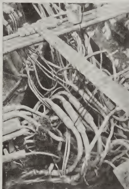
S. E. Corner Broadway and Houston Streets. Telephone Cables Exposed During Reconstruction of Manhole.
