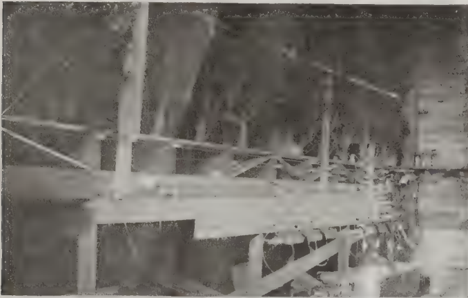
The Extemporized Switchboard: Simple but Sufficient
