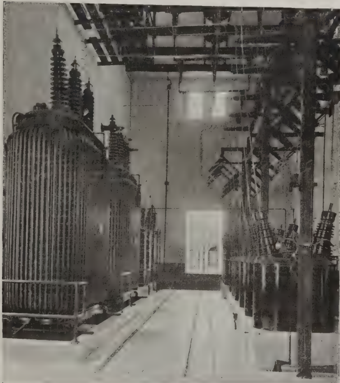
2 2500 kv.-a. 3-phase 100,000 to 2300v. Transformers and Oil Switches in Morel Substation
