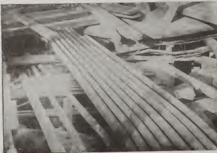
S. E. Corner Broadway and Canal Streets. 24-duct subway above; 16-duct below.
