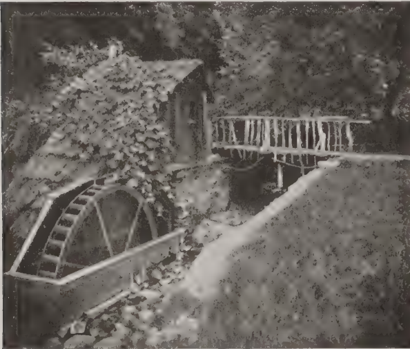
An overshoot wheel in a country estate. With flow of 0.35 cu. ft. per sec. in average weather, the "Fitz" wheel, 10 ft. in diameter and 1 ft. wide, generates enough power to supply 8 or 10 lamps at a time for several hours a day.
