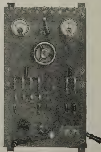
BATTERY CHARGING AND GENERATOR PANEL.
