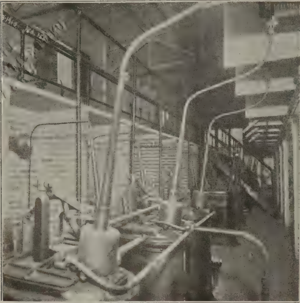
FIG. 5. HIGH TENSION SWITCH ROOM.
