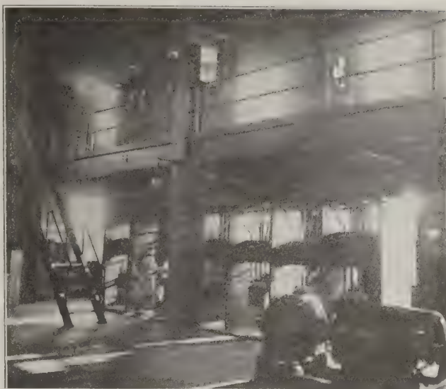
FIG. 3. BUS STRUCTURE AND SWITCHBOARD GALLERY, AUGUSTA STATION (WEST PLANT).
