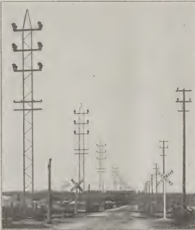
FIG. 7. 66,000-VOLT FLEXIBLE STEEL POLE LINE, AND 33,000-VOLT WOOD POLE LINE.
