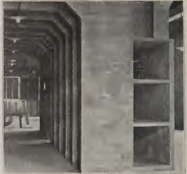
FIG. 7. COMPARTMENTS FOR 44,000-VOLT BUS IN TRANSFORMER HOUSE—6,600-VOLT OIL SWITCHES IN REAR.
