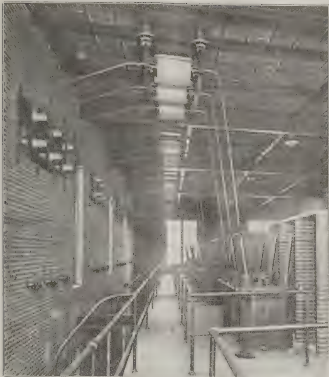
FIG. 15. 33,000-VOLT ENTRANCE AND OIL SWITCHES, LOCATED ON SECOND FLOOR OF JOPLIN SUB-STATION.
