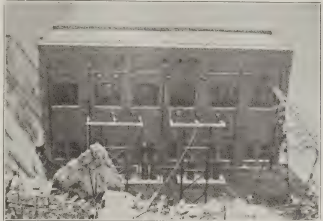
FIG. 9. NORTH END OF STATION SHOWING OUTGOING LINES LEAVING HIGH TENSION ROOM, LIGHTNING ARRESTERS SHOWN AT SIDE BELOW.
