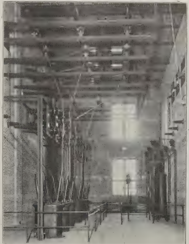
FIG. 11. 66,000-VOLT ROOM IN JOPLIN SUB-STATION.
