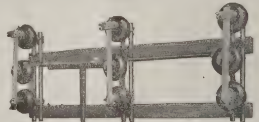
FIG. 2. TRIPLE POLE, 22,000-VOLT POLE TOP SWITCH.
