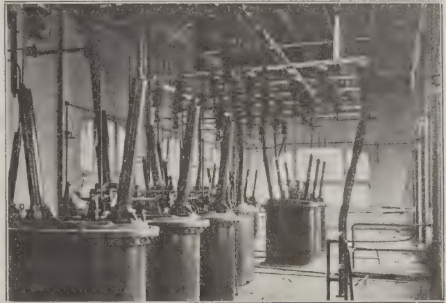
FIG. 5. VIEW OF HIGH TENSION ROOM.
