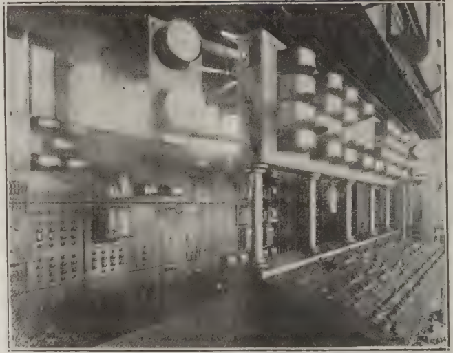
FIG. 5. CONTROL BOARD AT BLEWETT STATION.
