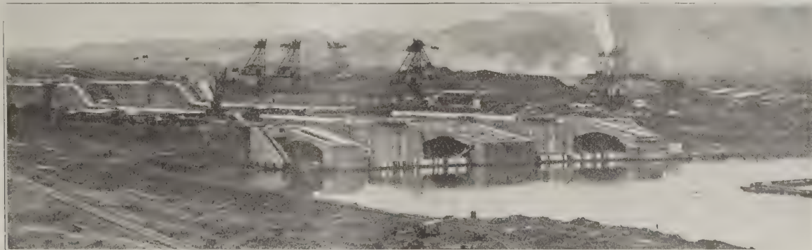
FIG. 1. THE GATUN LOCKS. A GENERAL VIEW LOOKING SOUTHWEST, SHOWING NORTH END OF LOCKS WITH TEMPORARY COFFER DAM IN PLACE.
