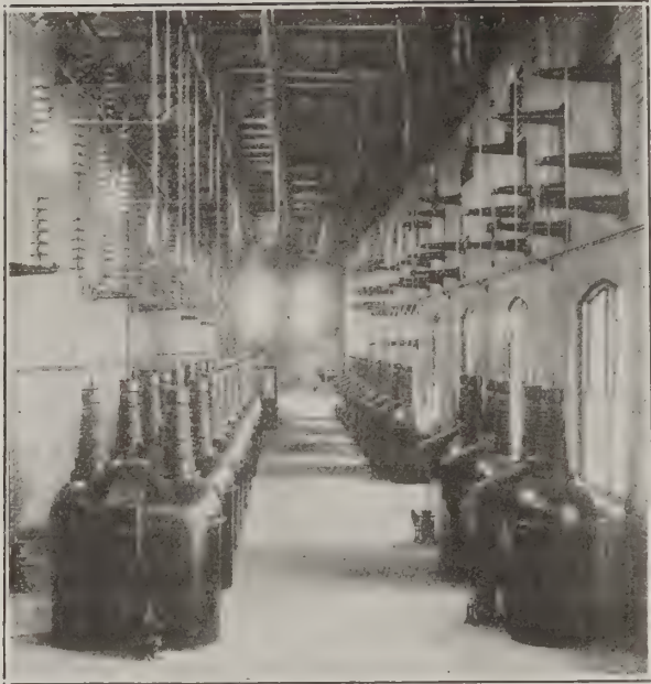
FIG. 3. HIGH TENSION SWITCH GALLERY AT BLEWETT PLANT.
