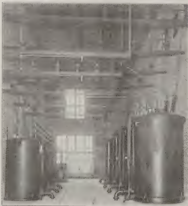
FIG. 12. TRANSFORMER ROOM IN JOPLIN SUB-STATION.
