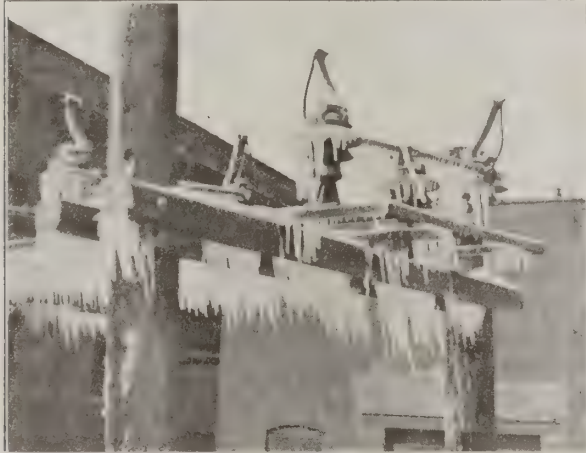
FIG. 1. THREE-PHASE HIGH TENSION SWITCH UNDER SEVERE ICE CONDITIONS.
