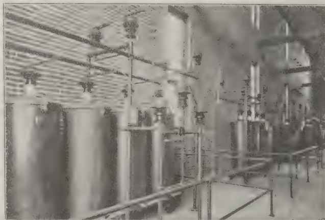
FIG. 14. 33,000-VOLT LIGHTNING ARRESTERS IN JOPLIN SUB-STATION.
