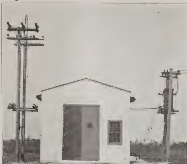
FIG. 6. SHOWING ENTRANCE TO AND LINES LEAVING MILL HAVEN SUBSTATION SERVING FACTORY DISTRICT.
