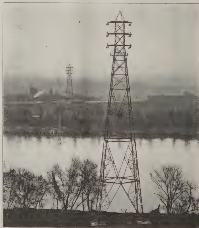
FIG. 10. TRANSMISSION LINE CROSSING TENNESSEE RIVER AT CHATTANOOGA ON 150-FOOT TOWERS—SPAN 1486 FEET OF 350,000 CIR. MIL. CABLE.
