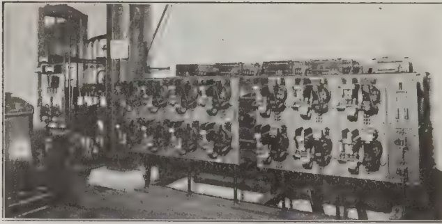
FIG. 8. CONTROL SWITCHBOARD FOR 1600 HP. MOTOR.
