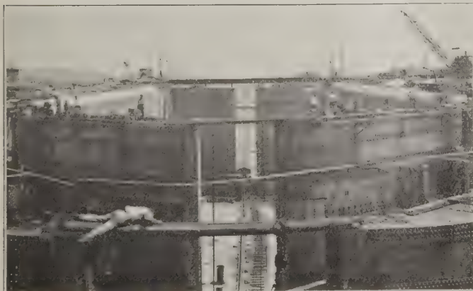
FIG. 2. GATUN UPPER LOCKS, WEST CHAMBER, LOOKING NORTH, SHOWING CONSTRUCTION OF THREE SETS OF GATES.
