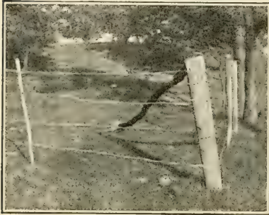
Figure 123.—A poorly-braced corner post from which it is impossible to stretch wires that will remain tight.
