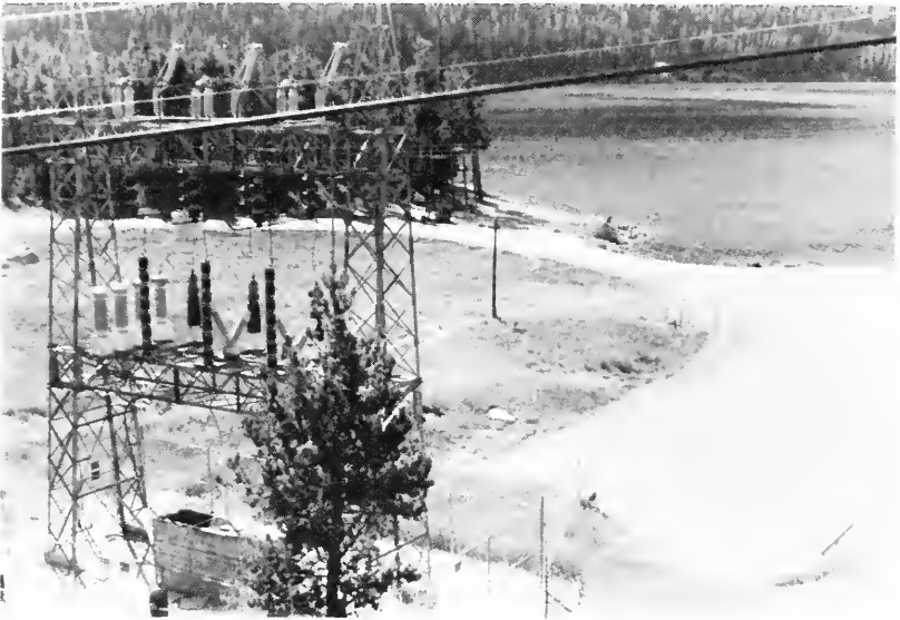
Fig. 1 Adams tunnel gate house site with photographer facing south toward Grand Lake. Intake structure and conduits to gate house are buried under paved roadway and parking area at the right side of the picture. Photo by G.F. Price.
