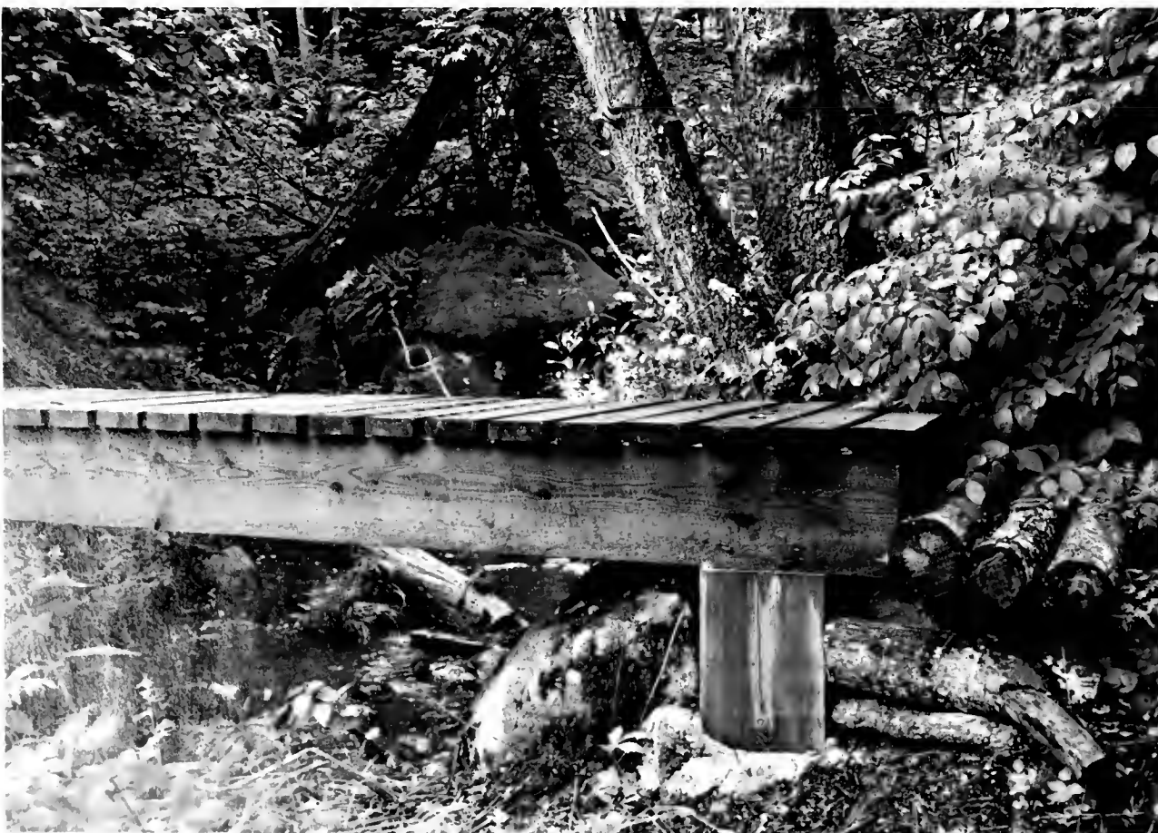
1. Wooden bridge near La Cabanasse (42.504° N; 2.130° E; 1400 m altitude) infested with elm beetles in June 2008. Photo: Theodoor Heijerman
