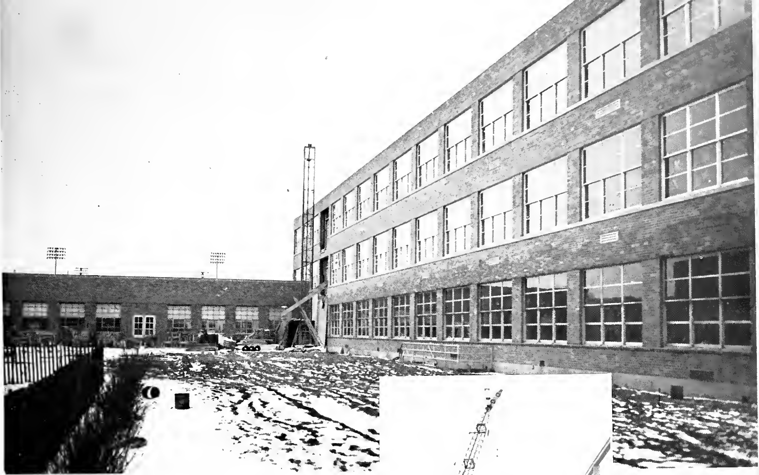
Construction progressed but many difficulties prevented use of the classrooms until fall.
