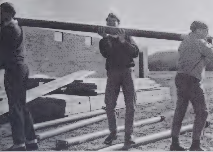
Jimmy Kent, Danny Stansell, and Gary Ball help in building the field house
