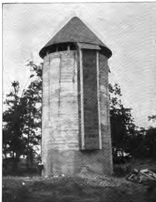
FIG. 403. WING CEMENT SILO.
