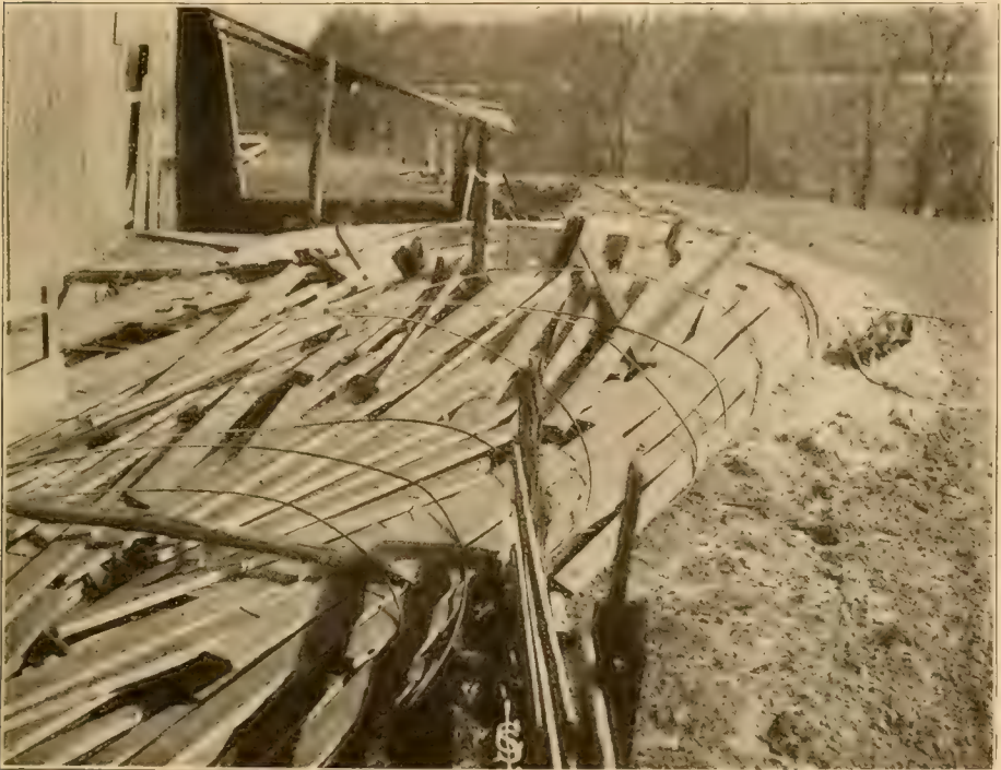
Fig. 15.—A Silo Which Was Not Properly Anchored, after a Storm.
