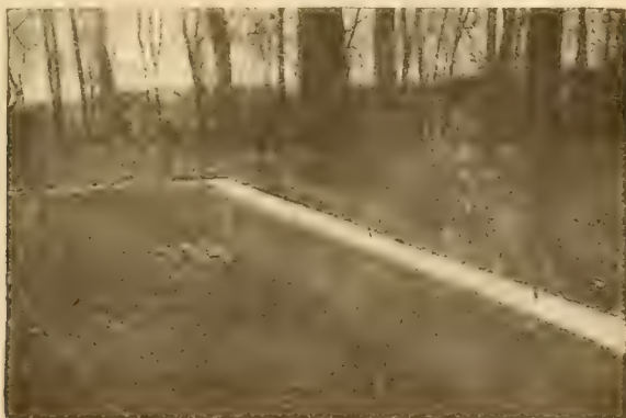
Fig. 20.—Foundation Wall for a Small Shed. Showing Bolts for Attaching the Wooden Sill to the Concrete Foundation.
