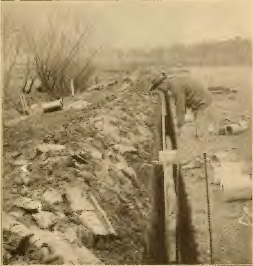
Figure 10.—Laying 6-Inch Tile In a 4½-Foot Trench. The man standing at the side of the trench is laying tile with a tile hook. Courtesy of the Wisconsin Experiment Station.
