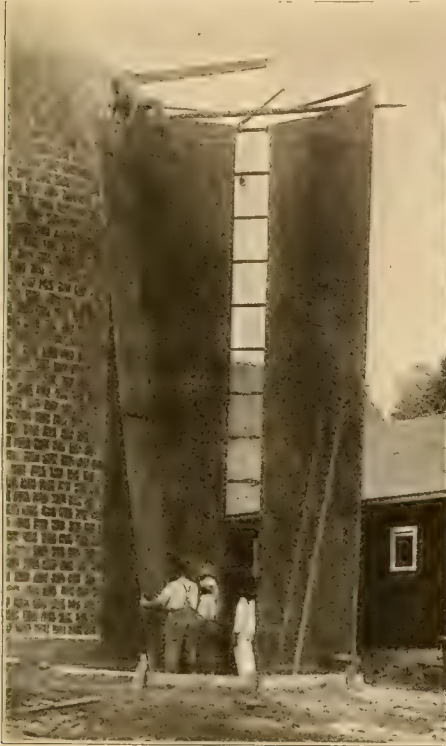
Fig. 11.—Erecting a Stave Silo without scaffolding. Door frame in place and raising staves. Courtesy of the Iowa Experiment Station
