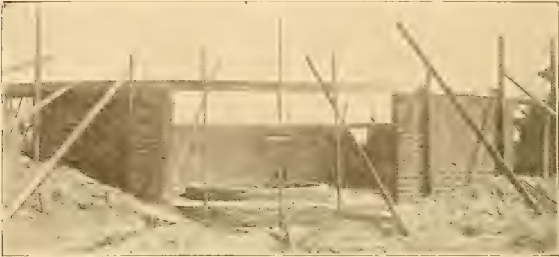
Fig. 19.—First-story Wall and Foundation for Silo, Feed Alley and Manger; Sill in place, ready for joists and studs.
