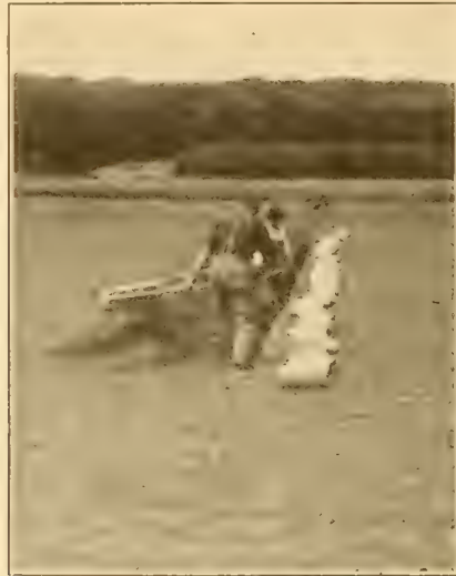
Fig. 7.—Trenching for Tile. Note the line necessary. Only the unskilled workman will attempt to get the ditch straight enough without a line. Courtesy of the Minnesota Experiment Station.
