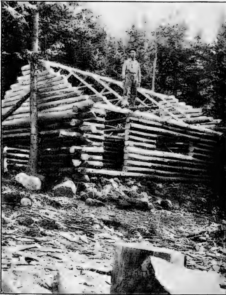
FIG. 3.—A summer home on Cheyenne Mountain, Colo., being constructed from aspen logs. These trees were cut within a radius of 200 yards of the structure. Elevation at this point, 9,000 feet.
