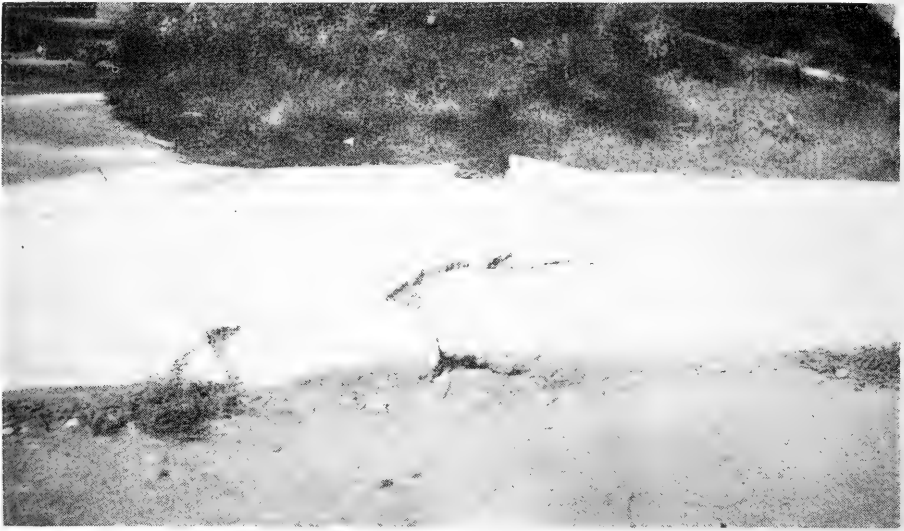
FIG. 146. Defective concrete walk.
