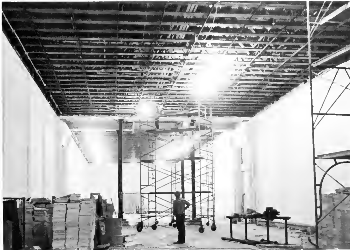
At left, workmen complete the steel framework for the renovation of Hall 18. The hall's new ceiling provides the flooring for new working space on the third floor, formerly this space was a light well. The new space is to be used for offices and laboratories in the Division of Insects, and for major storage areas and a lecture/class room for new educational programs.
