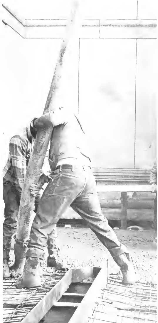
A section of the north portico gets a new base as fresh concrete is hosed in. As part of the Museum's rehabilitation program, storage areas currently under the portico and front steps will be converted into administrative office space.
