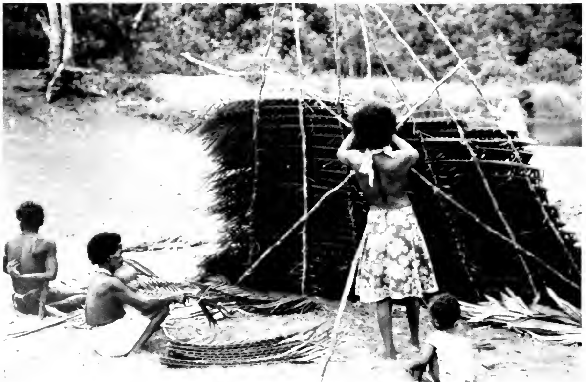
An Agta woman constructs her family's lean-to shelter. A relative helps her by fashioning palm fronds into shingles.
