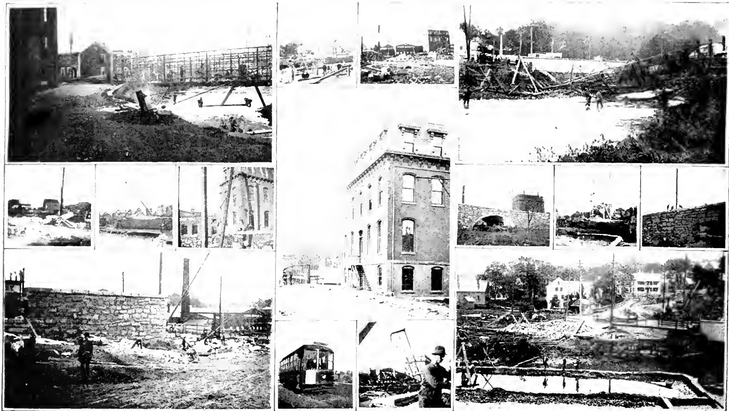
ABOLITION OF THE GRADE CROSSING AT PUTNAM STREET, SHOWING WORK AT DIFFERENT STAGES.
