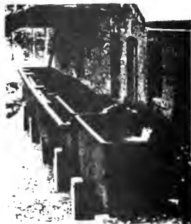
Fig. 29. Filtering arrangement of a hatch house. Front, 2 pre-filters, behind 3 filters.
