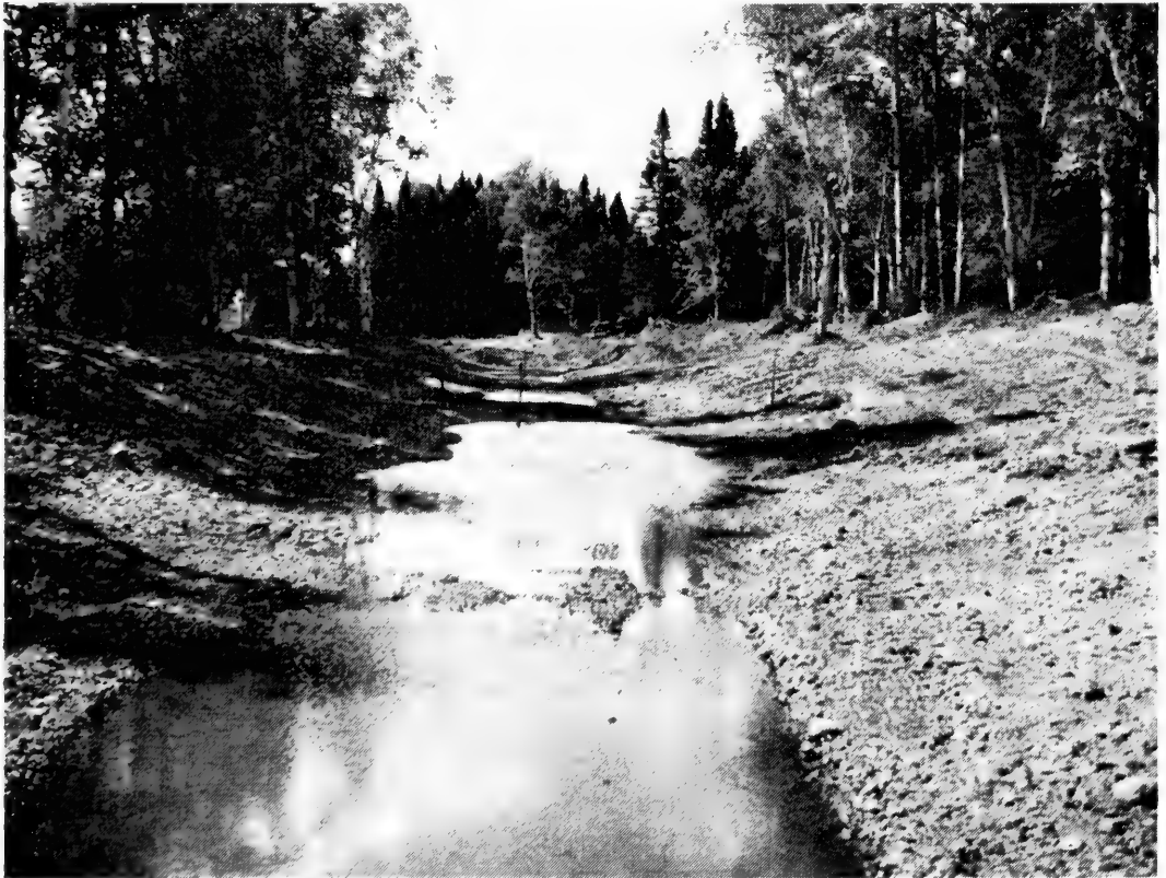
Early construction stages of an artificial spawning area for Atlantic salmon on Indian River. This is associated with an hydroelectric water diversion.
