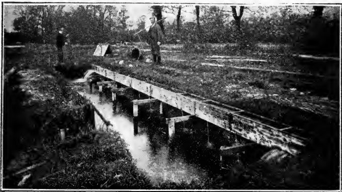
AN OVERHEAD HORIZONTAL BOX SCREEN.
