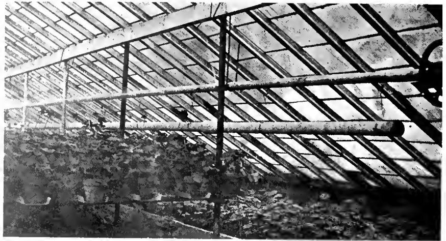
Wittbold Watering Device—Spraying a Center Bench from a Side Pipe Line.
