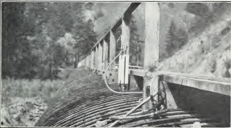
FIG. 3.—MERCURY MANOMETER AND FLUORESCIN GUN (GAUGE 1) ON 13½-FOOT PIPE OF NORTHWESTERN ELECTRIC CO., WASHINGTON. (No. 52.)
