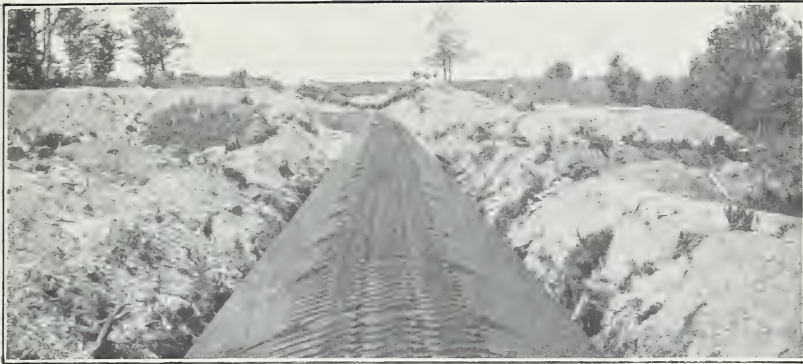
FIG. 1.—TRUNK LINE, SALMON RIVER POWER CO., NEW YORK. TAKEN ON REACH TESTED. Typical alignment. Straight in profile. (No. 51.) See figure 2.
