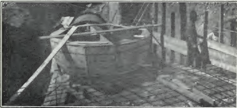
FIG. 2.—FORM FOR BOWL, FLOOR REINFORCEMENT, AND CAST-IRON PIPE FOR INLET SECTION FOR STRUCTURE IN FIGURES 1 AND 3.
