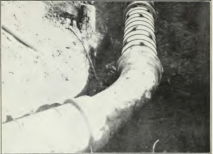
FIG. 1.—EVEN WITH 27 CAST-IRON BENDS LIKE THIS THE ASTORIA, WASH., PIPE SHOWS A CAPACITY 17 PER CENT MORE THAN THE AVERAGE. (No. 23.)
