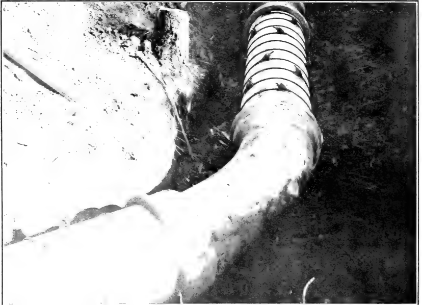
FIG. 1.—EVEN WITH 27 CAST-IRON BENDS LIKE THIS THE ASTORIA, WASH., PIPE SHOWS A CAPACITY 17 PER CENT MORE THAN THE AVERAGE. (No. 23.)
