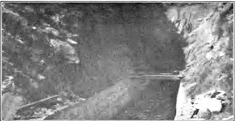
FIG. 2.—VIEW TAKEN FROM STRUCTURE IN FIGURE 3. Hillside cut ravelings enter pipe and reduce capacity. A condition to be avoided.
