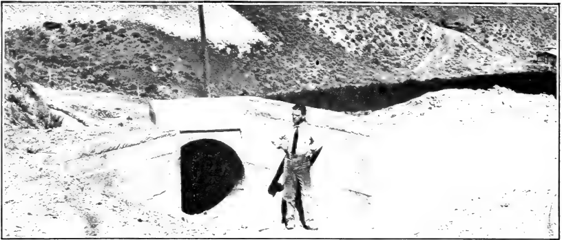
FIG. 1.—TYPICAL OUTLET STRUCTURE. WILL PARTIALLY RECOVER VELOCITY HEAD. Pipe is one-half diameter too high for inlet structure. Too much air would enter.
