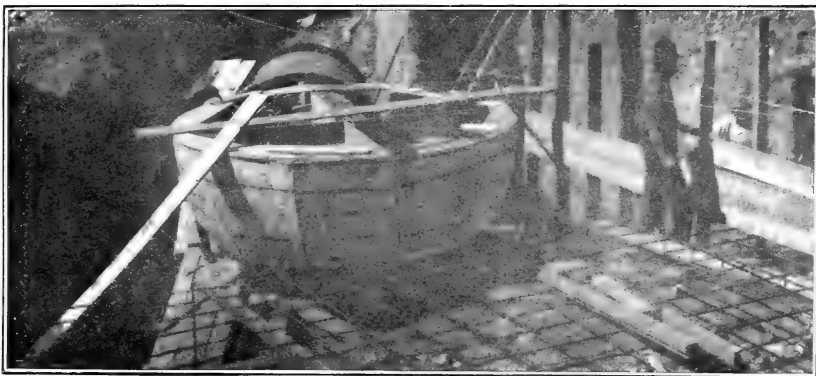
FIG. 2.—FORM FOR BOWL, FLOOR REINFORCEMENT, AND CAST-IRON PIPE FOR INLET SECTION FOR STRUCTURE IN FIGURES 1 AND 3.
