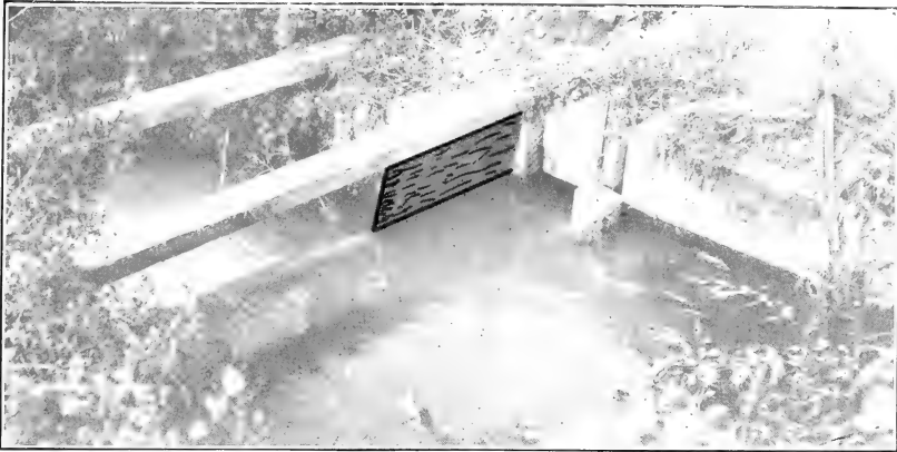
FIG. 1.—TYPICAL CIPOLLETTI WEIR, WITH HOOK GAUGE IN STILLING BOX. Note brush screen in foreground to reduce velocity of approach.
