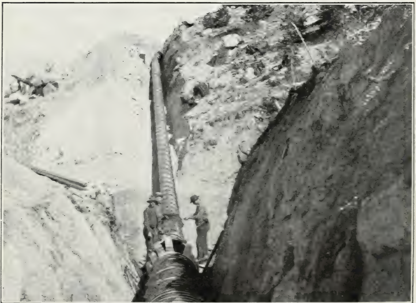
FIG. 2.—PIPE FOR BUTTE, MONT., MUNICIPAL SUPPLY. (No. 32.) SPRINGING IN A BUCKLE JOINT.
