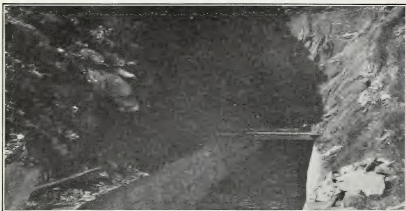
FIG. 2.—VIEW TAKEN FROM STRUCTURE IN FIGURE 3. Hillside cut ravelings enter pipe and reduce capacity. A condition to be avoided.
