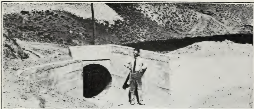
FIG. 1.—TYPICAL OUTLET STRUCTURE. WILL PARTIALLY RECOVER VELOCITY HEAD. Pipe is one-half diameter too high for inlet structure. Too much air would enter.
