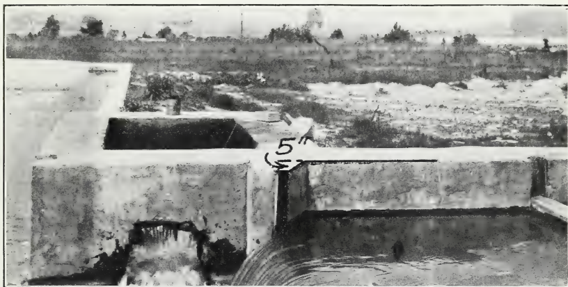
FIG. 2.—WEIR AT OUTLET OF PIPE NO. 30, NORFOLK COUNTY WATER CO., VIRGINIA. The immediate bottom contraction similar to that shown at side, although water above weir wall is several feet deep.
