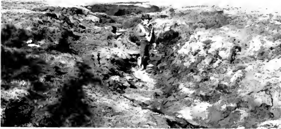
Figure 36. Upstream view of thermal and fluvial erosion in the access road at Ugnuravik River, acting as a long-term sediment source to the river.
